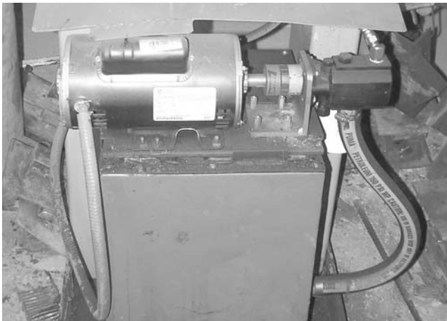
This view shows a close up of the Motor, Pump and Tank
